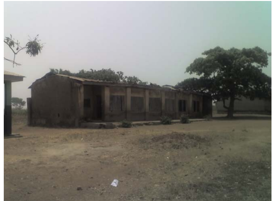
Unsafe classroom building
