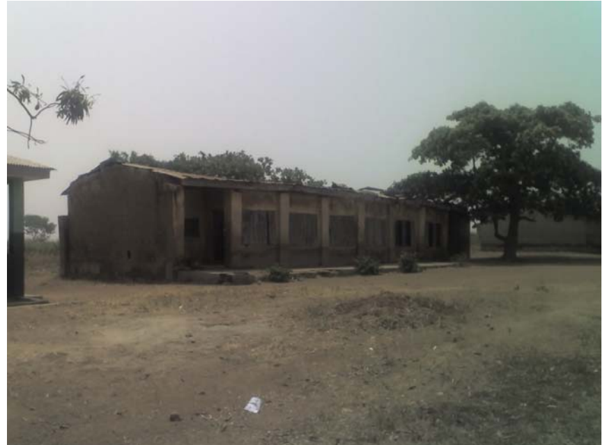
Unsafe classroom building
